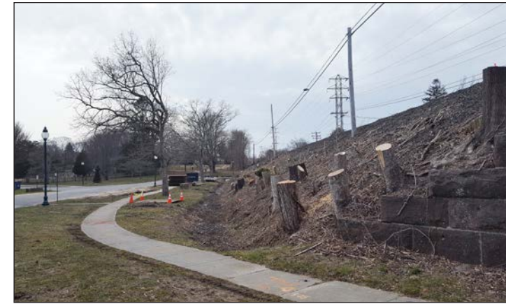
All vegetation has been removed within the LIRR right of way along Hook Mill Ln. Village government reportedly will have some input on re-vegetation.
